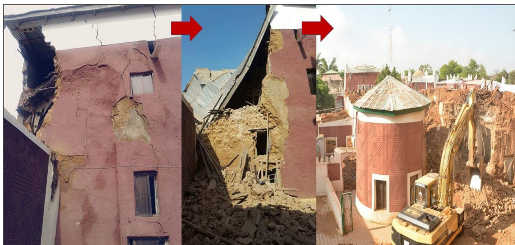
Figure 8. The Emir's wing self-collapse and demolition process after attaining ageing and limit of repair
